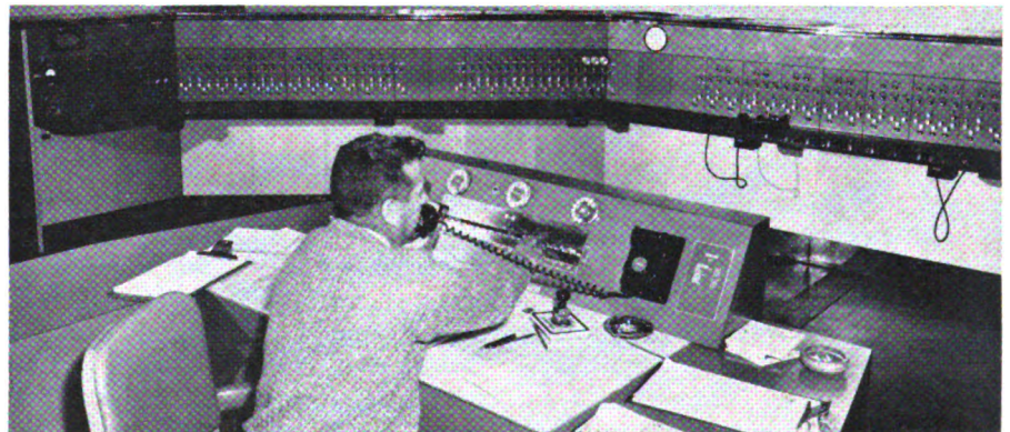
Gwelo CTC machine controls 182 miles of line between Gatooma and Heany Jct.
