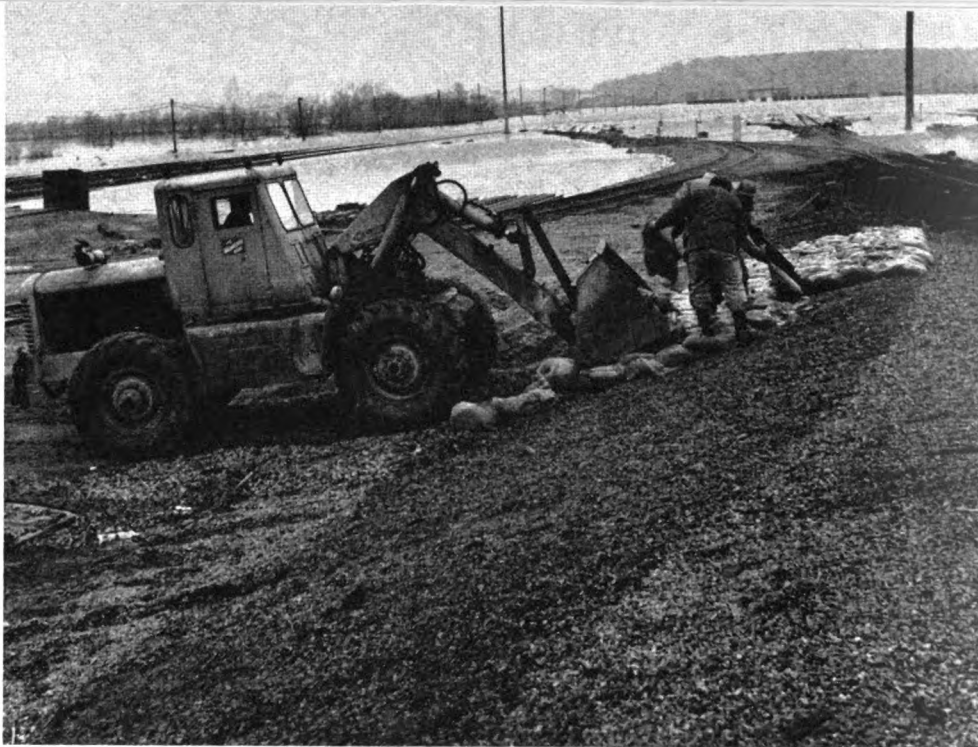
Sand bags were placed along side of the hump to prevent water from washing away soil and ballast. Here is removal of sandbags after water has receded.
