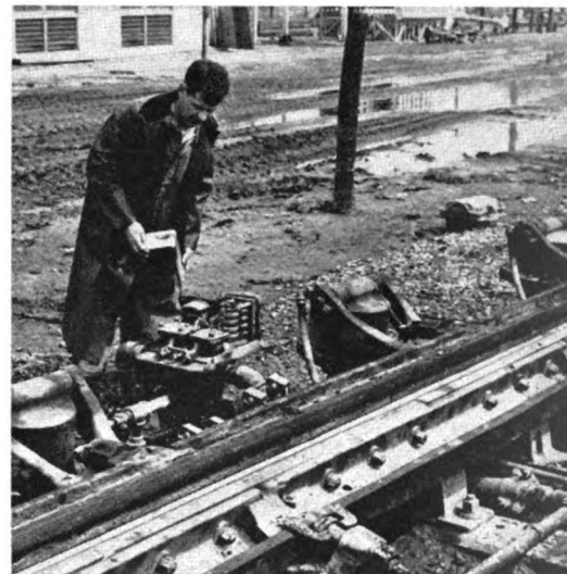
Retarder control valves are examined after water receded.
