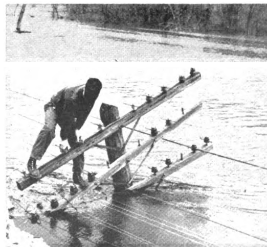
This pole line did not escape high flood waters.
