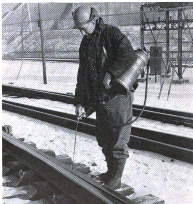
Wayne Davis, leading signal maintainer, uses garden weed spray for spreading graphite switch plate lubricant.
