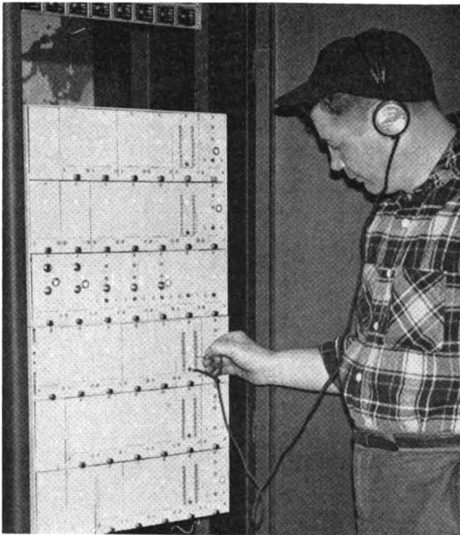
D. E. Bissell, signal mechanic, checks out solid state units by listening to audio tones with a headphone.
