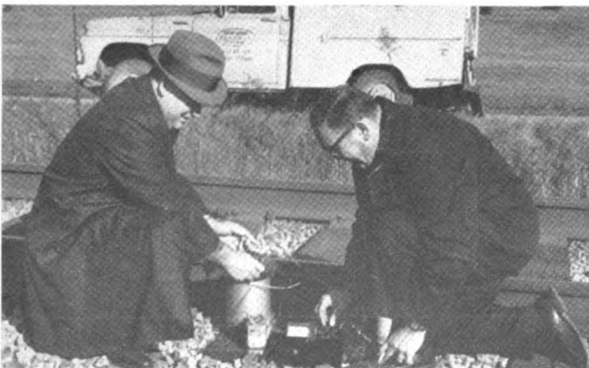
D. W. Shackley (left) and J. D. Rock check battery voltage to solid state code transmitter used in track circuit test.
