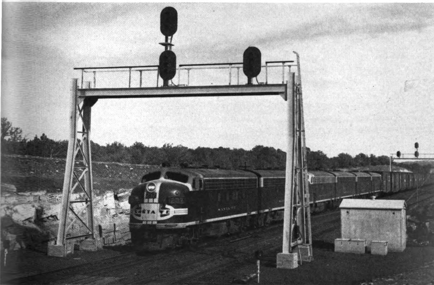
The work is done and the trains are rolling over 44 miles of new double track, CTC controlled for reversible running.
