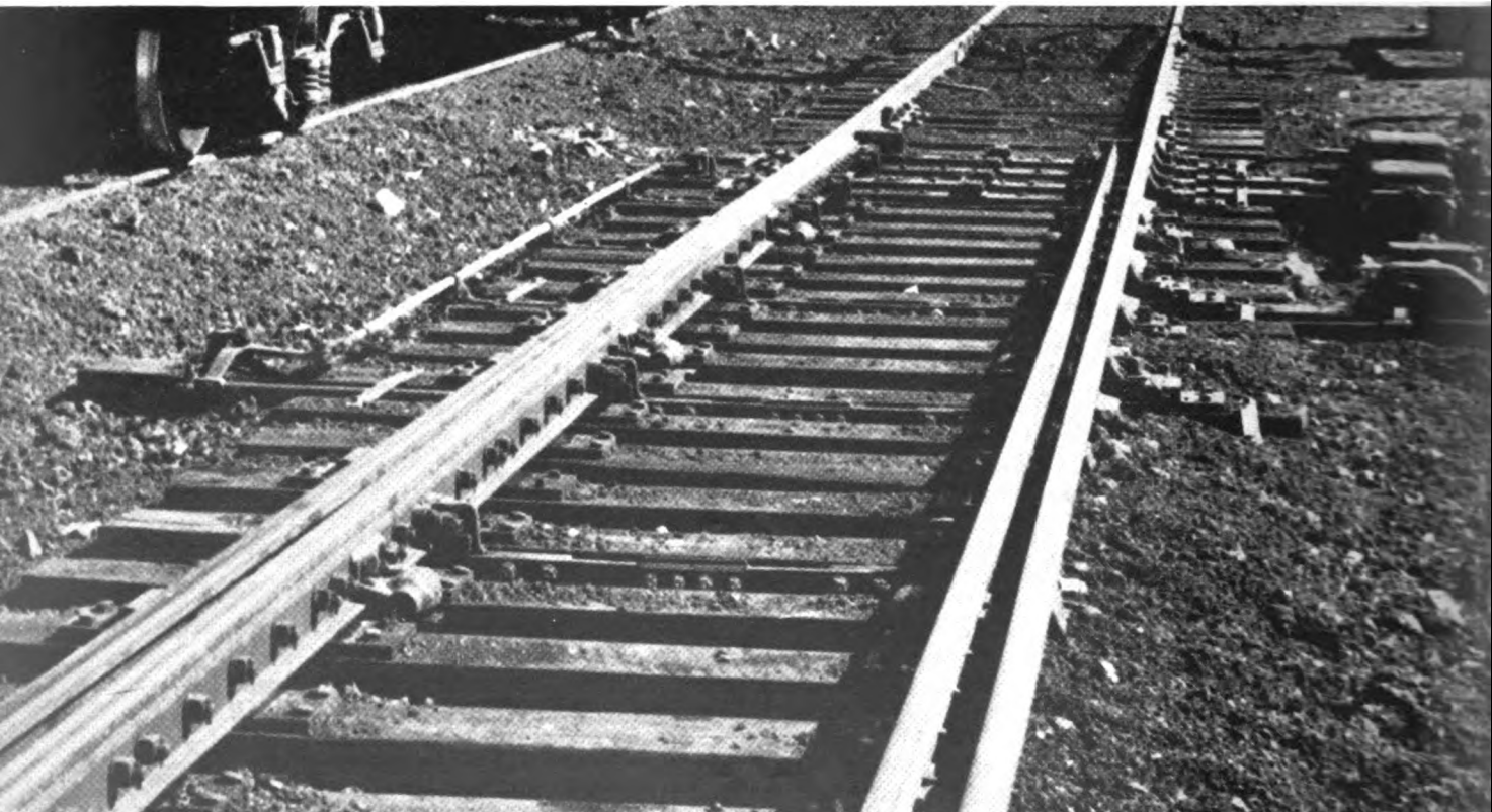
A circuit controller is attached to the #5 rod of the 39 ft points to check that the entire point has been fully thrown.
