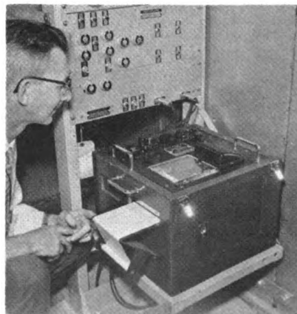
▲ Pengraph recorder and test panel at the hotbox detector location aid maintainer in detector preventive maintenance.
