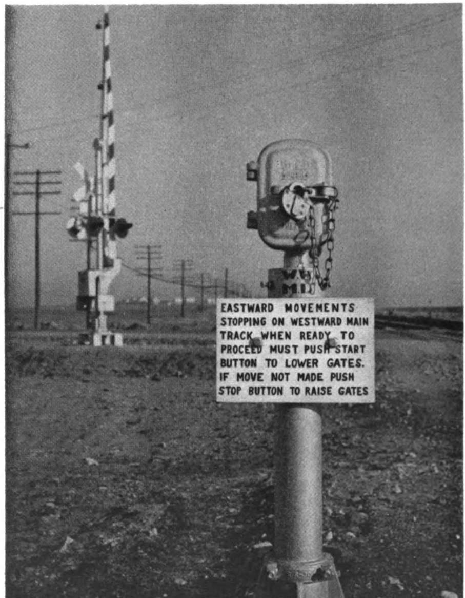
Pushbuttons are provided to lower and raise gates for reverse moves. This view is looking east toward the Midland avenue crossing.
