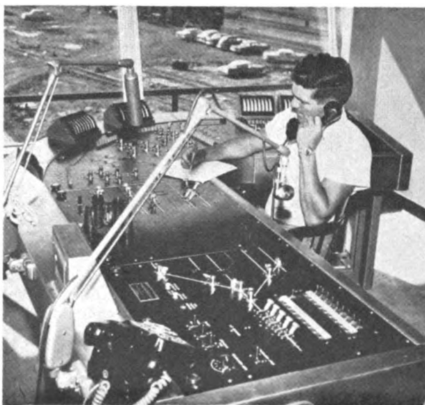
Retarder operator monitors the classifying process. GRS Class-Matic system provides automatic operation of retarders and class track switches. Indicators tell operator how many cars are in each class track.
