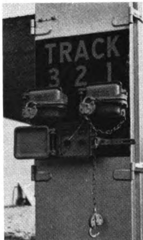
Switching crew can take manual control of gates when they are working near, but not over the crossing. Each track has its own "raise" and lower pushbuttons.
