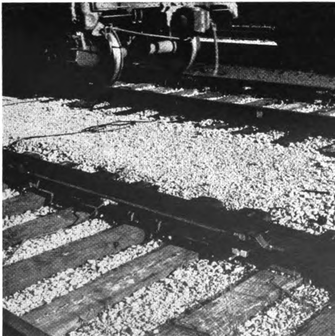
FLANGE TREADLES, on the hump lead and each body track, are clamped to the rail base. This mobile lab installation was developed by General Railway Signal Co.,
