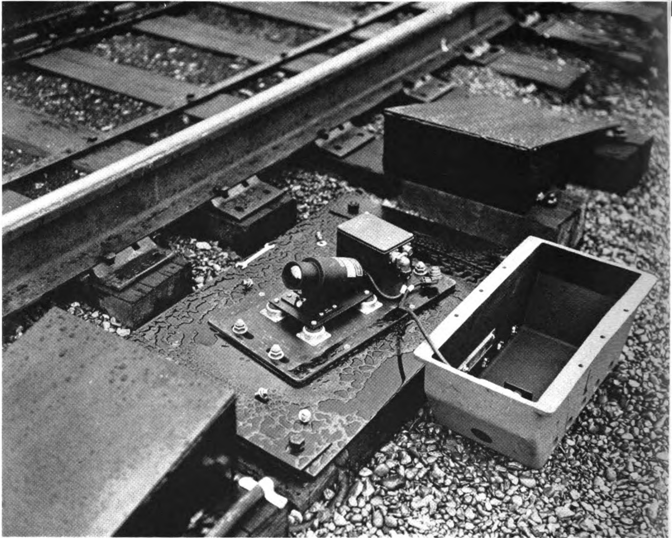
Hot box detector, tilted upward at an angle, views journals from bottom to top as they recede.
