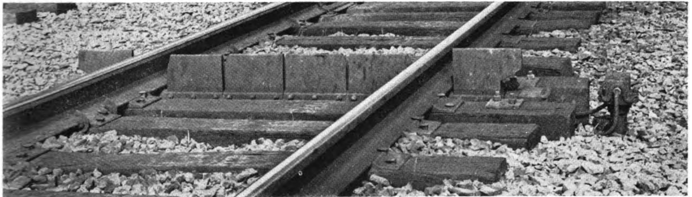
This dragging equipment detector is self restoring. The Southern Installed six of these safety detectors in a 150-mile CTC project.
