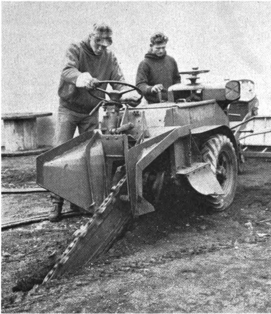
Cable was trenched in using this model 702 ditcher and a tractor with a back hoe
