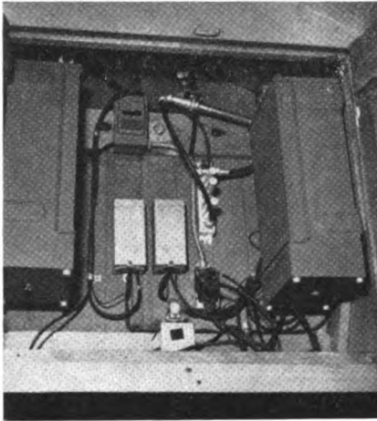
Base station radio equipment is the single-package type operating on 117-volts a.c.
