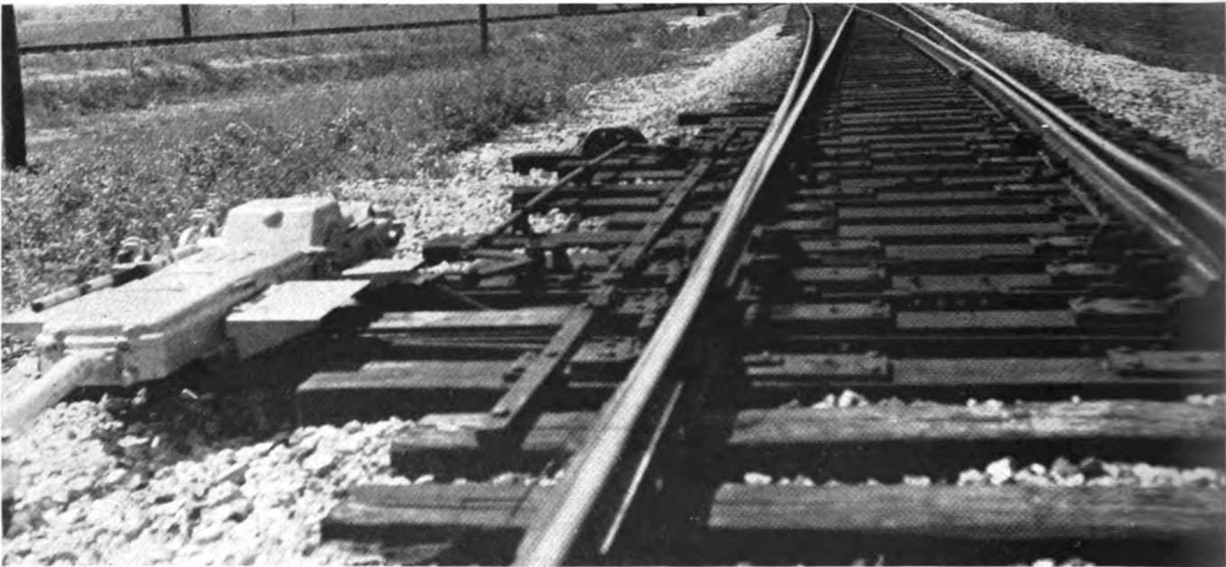
Power switch at east end of siding at North River. The long switch points require a helper rod to the mid-point.
