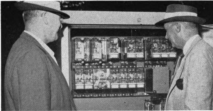
Maintenance Foreman L. W. Davidson (left) and Signal Supervisor C. Westberg look at Trakode (slow coding principle) equipment in Pilgrim instrument case
