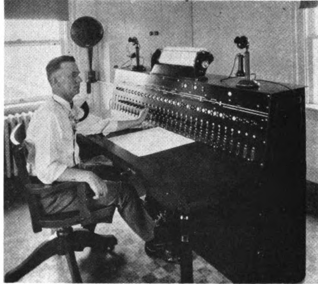
This is the control machine for first centralized traffic control installation; on the NYC in 1927
