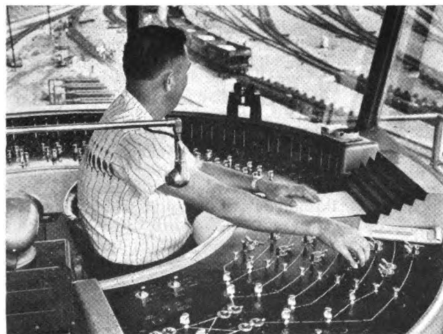
Track-fullness indicators are included on panel of "monitor" machine in automatic retarder yards
