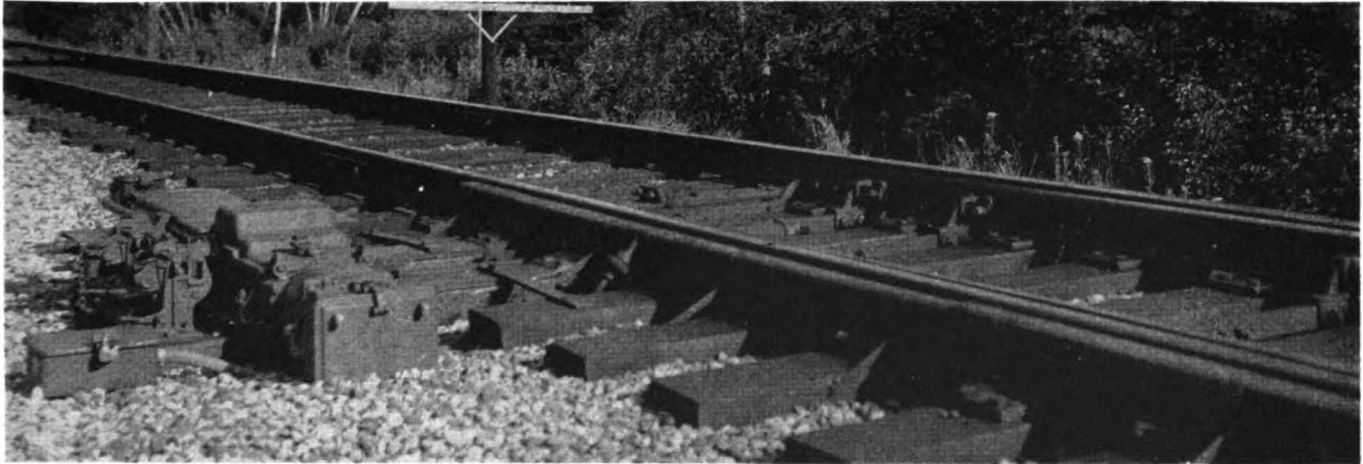
Gas heaters, controlled by CTC, melt the snow and ice in switches
