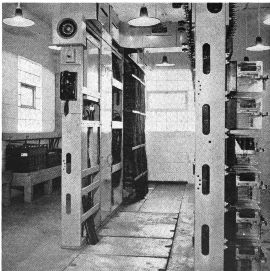
Talk-back speaker in sub-tower relay room connects to Hayford tower operator
