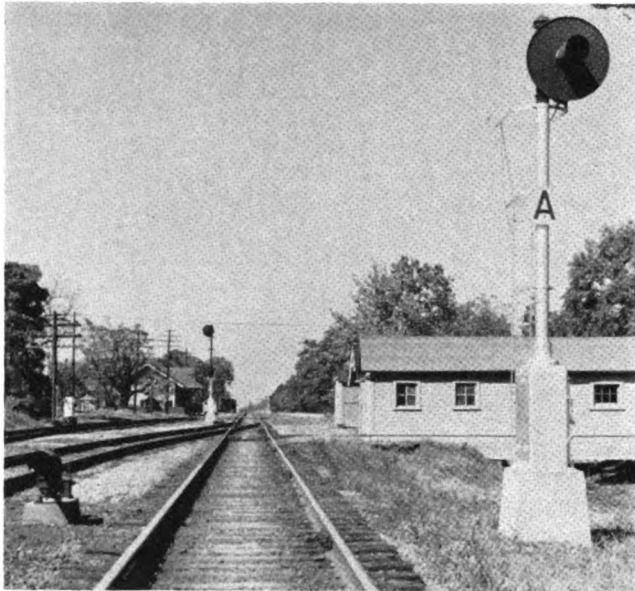
L&N provides complete signaling at power switches in full CTC with dwarf for siding and high signal for main track
