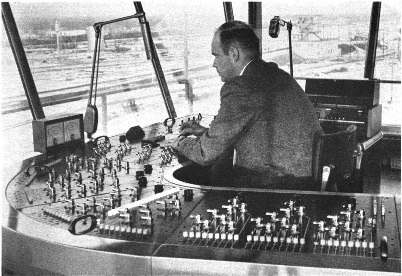
Track fullness is shown by line of lights (by operator's elbow) on retarder control panel
