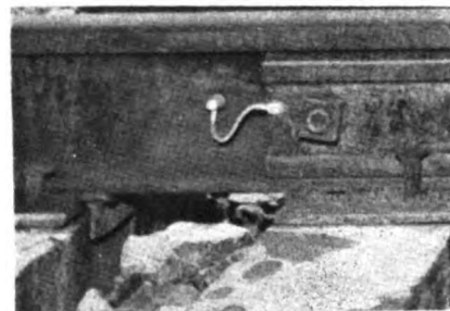
Special CN design bonds are on the gauge side of the rail and joint bar
