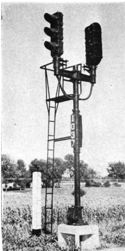
Double-track automatic signals have one head mounted to left of track it governs
