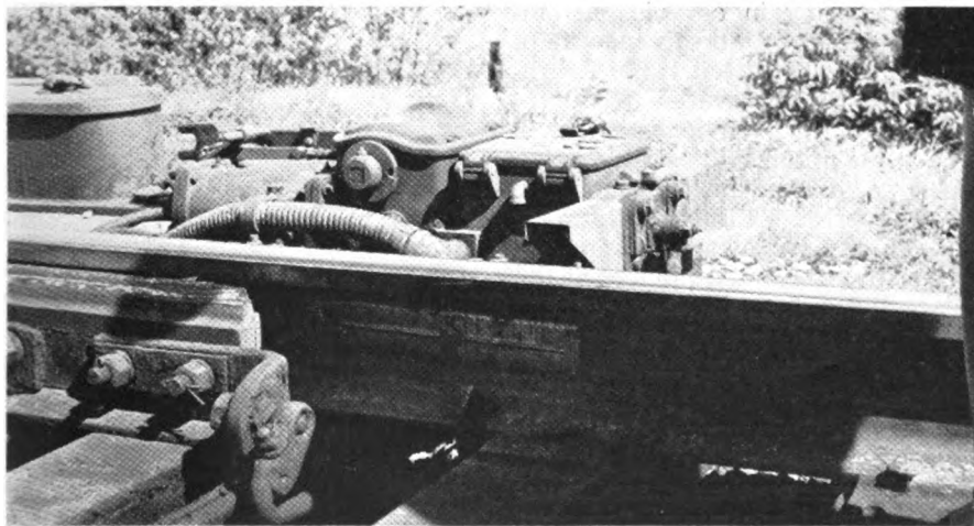
Snow melter coils, 1/4 in. thick, 3 in. wide and 15 in. long, are bolted to the gage side of web of rail
