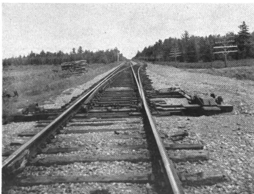
Spring switch has mechanical facing-point lock
