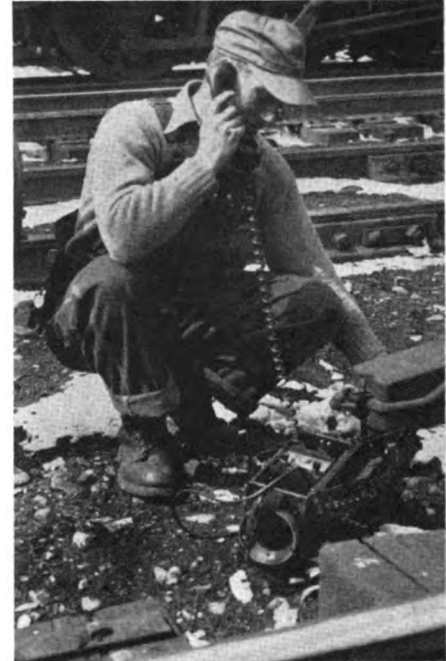
SIGNAL MAINTAINER has portable telephone to call interlocking operator in tower
