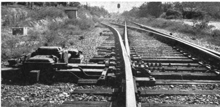
DUAL-CONTROL , low-voltage switch machines are mounted on two dapped ties
