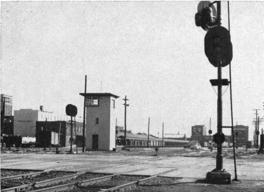
EIGHTH STREET CROSSING (looking east): colorlight signals No. 8 governing train movements in both directions over crossing are controlled from tower
