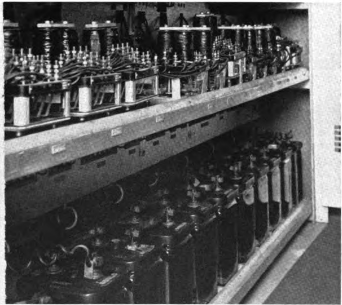
RELAYS AND BATTERIES in sheet-metal house
