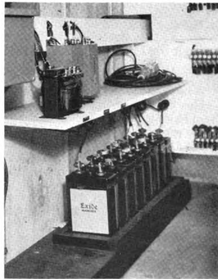
BATTERIES ARE IN instrument house
