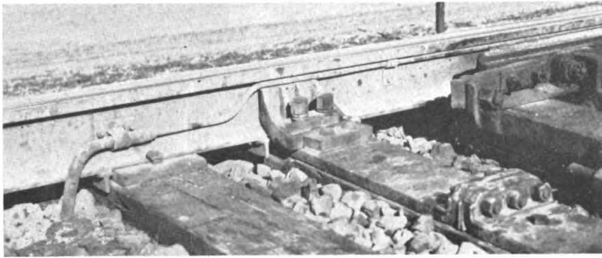
ELECTRIC SWITCH HEATERS are the so-called "rod" type
