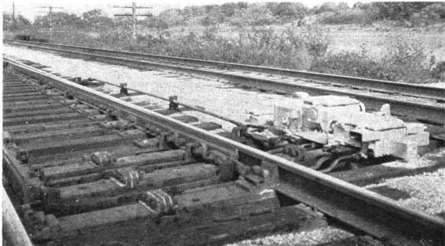
A HELPER is connected to mid section of the long switch points
