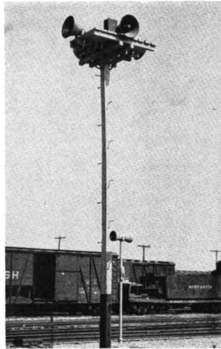
Pagers on elevated platform
