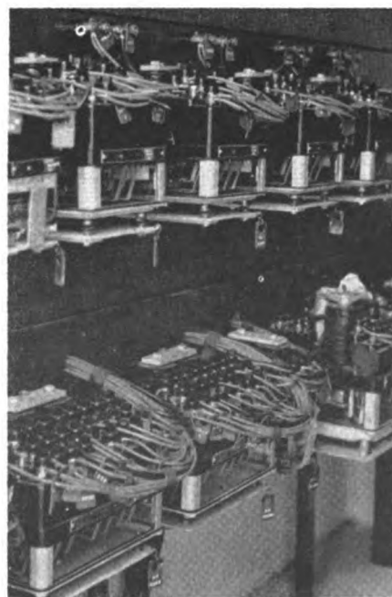
Conventional relays are wall-mounted
