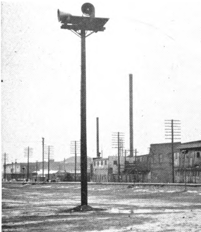
Paging speakers on platform on top of wood pole
