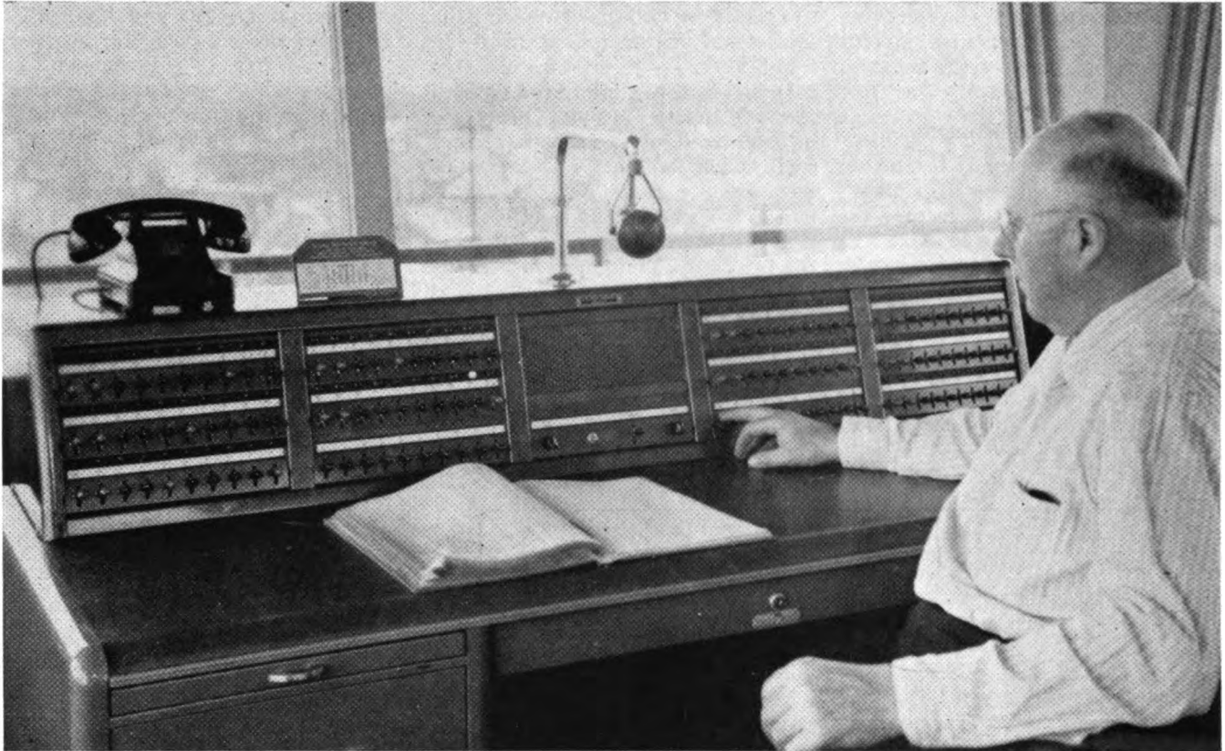
The communications control console is on the yardmaster's desk in an office on an elevated tower
