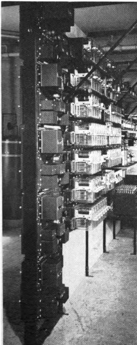
Narrow band and broad band control equipment in Milford relay room
