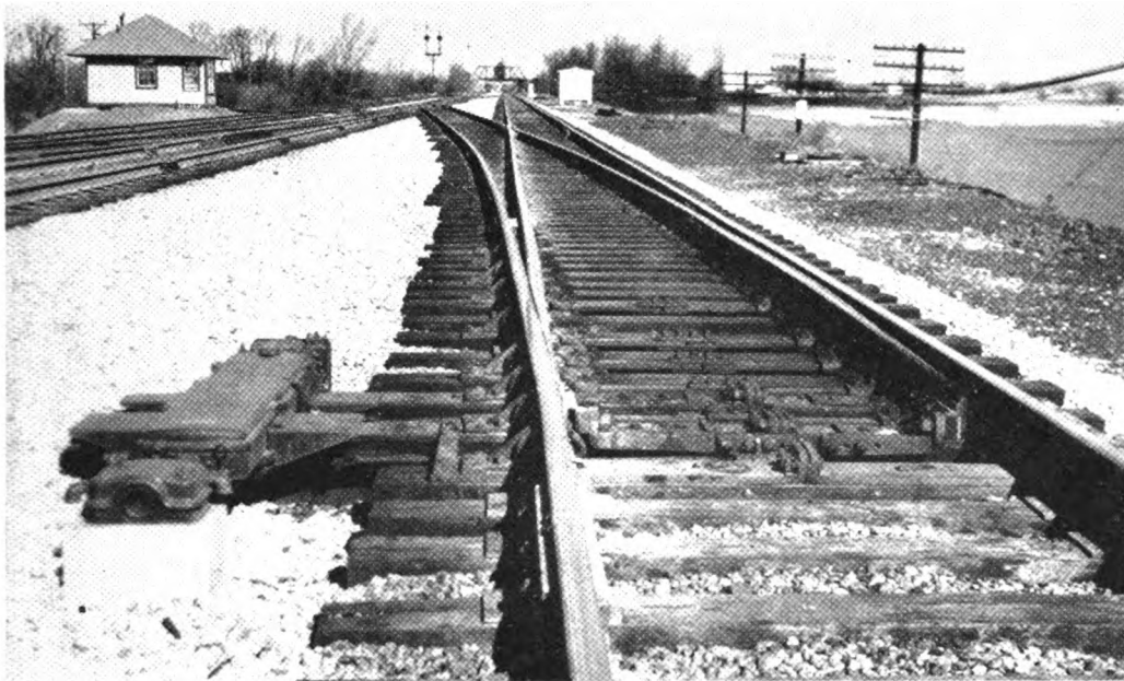
Left — Switches are operated by 32-volt high-speed machines Below — The new signals are the color-position - light type
