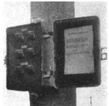
Case with push buttons for the control of crossing gates
