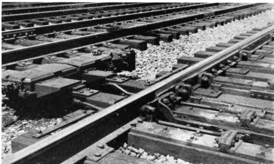
Power switches are well constructed
