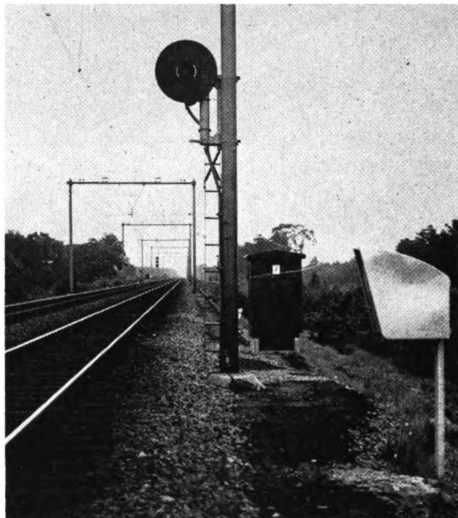
This is one of the automatic block signals near this new interlocking
