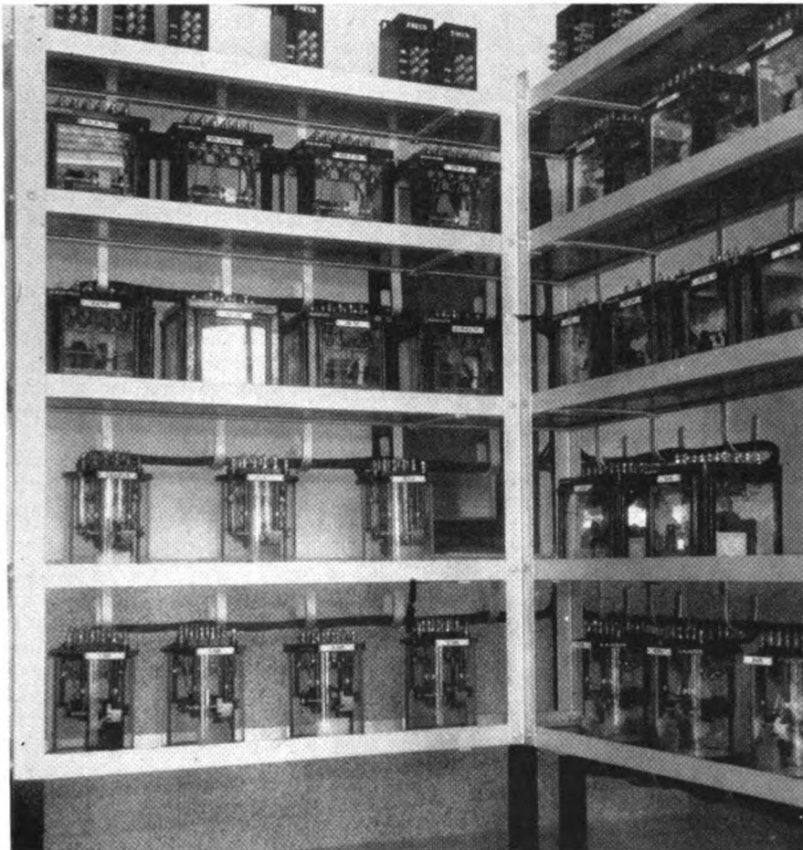
Metal hangers keep wiring straight on relay racks
