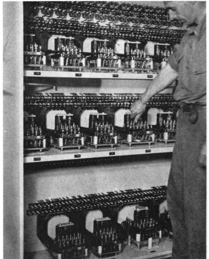
Relays and wiring, using No. 9 solid copper wire, were installed in cases while in the shop
