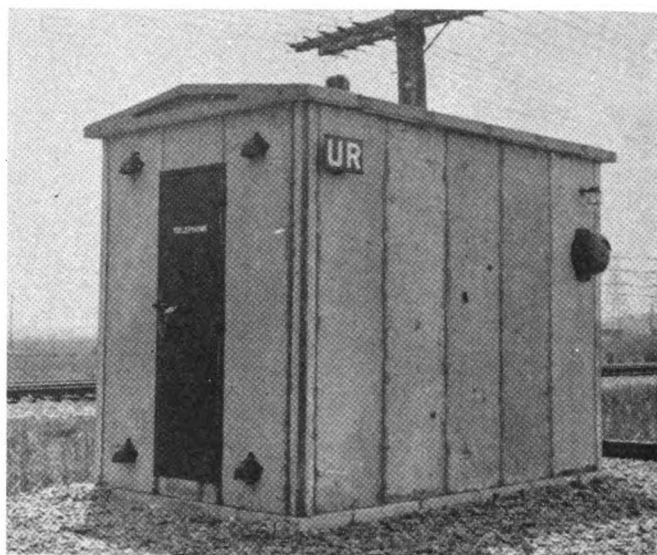
Pre-cast concrete sectional type of house for relays and battery at UR
