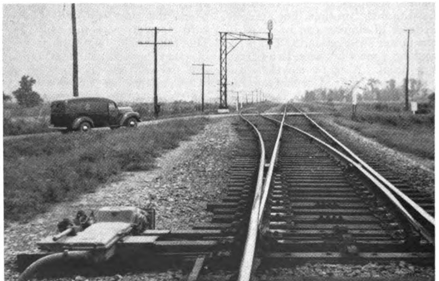
The switch machines are the dual-control type
