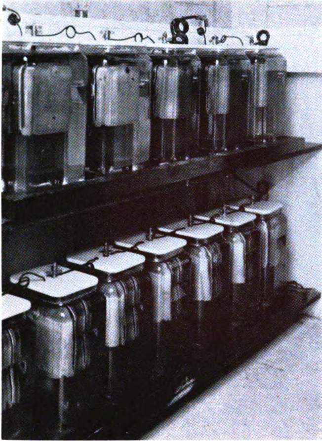
At each intermediate signal there is a set of 16 cells of 1000-a.h. primary cells which feeds coil and lamps
