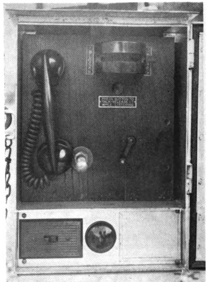
Phone box near end of tunnel includes toggle switch and the 2-inch red lens
