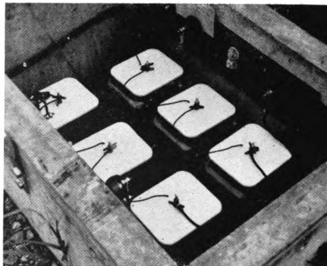
Edison primary battery is used to feed track circuits where no a.c. power is available
