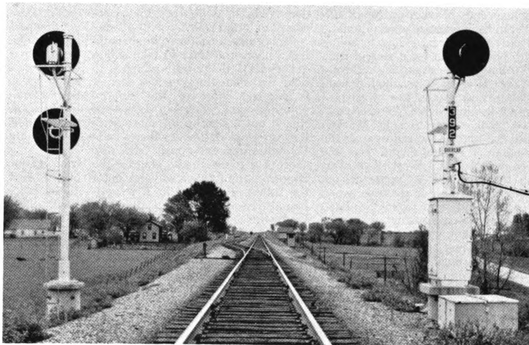
Typical head-block double signal location at the end of passing siding, note overlap sign on signal at right
