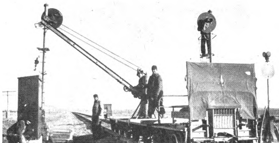
A crane on a motor car was used to erect the signals
