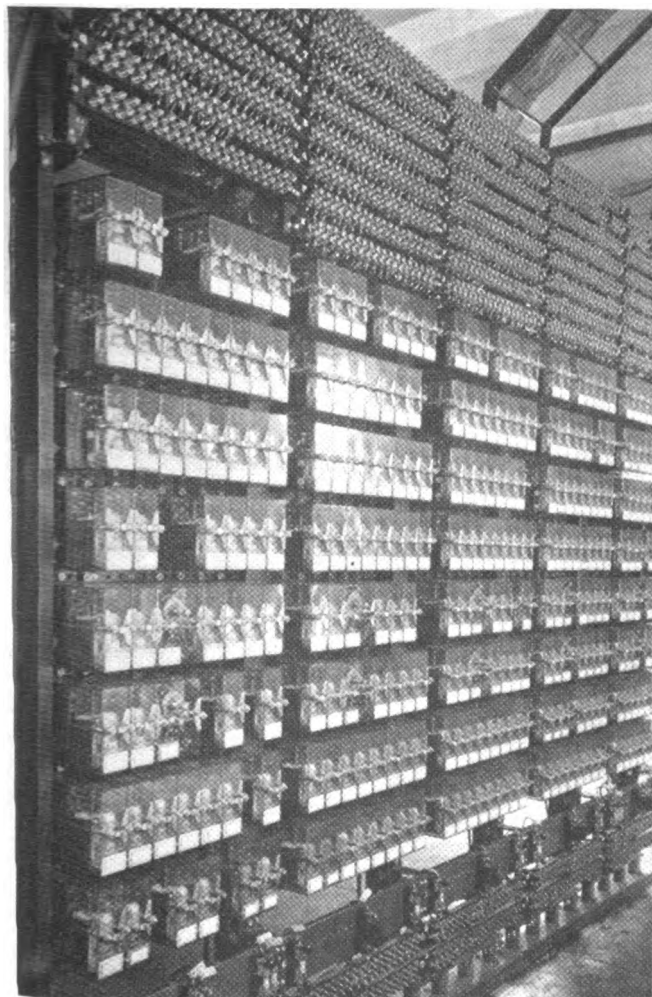
Plug-in relays in racks
