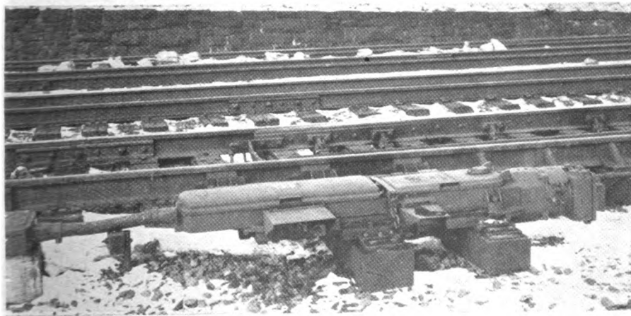
The new switch machines are the Model 5C
