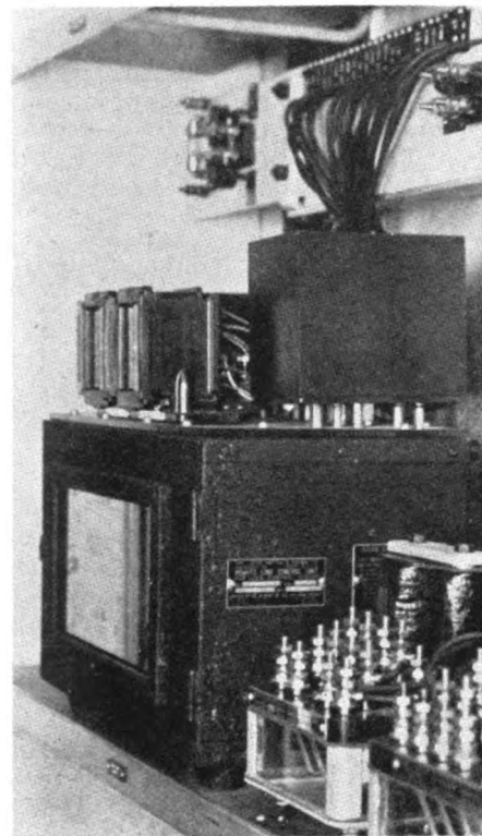
Carrier equipment at Lakeside
