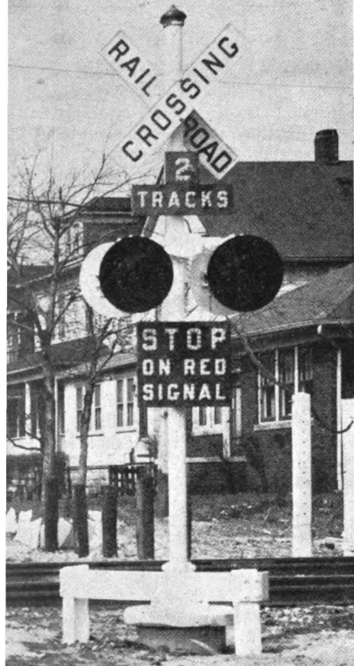
A typical flasher installation on the Wabash
