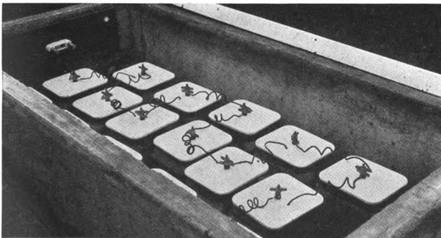
Primary battery in box at intermediate signal
