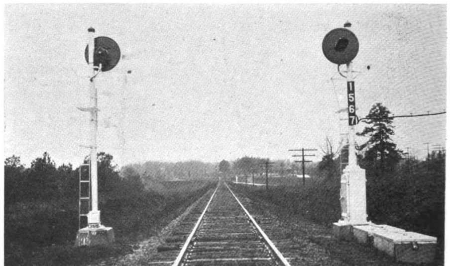
Intermediate location with battery boxes
