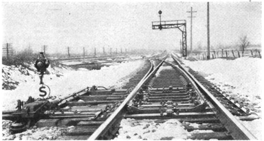
A spring switch at the east end of the siding at Leavittsburg
