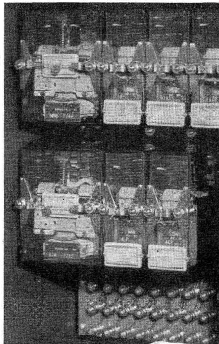
Left—Interior view of the field instrument case, showing plug-type relays, rectifiers, terminals, etc. Switch control relay is in upper right-hand corner. Below—Relays located in the rear of control machine
